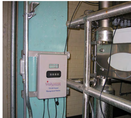
Sensor Management Station
