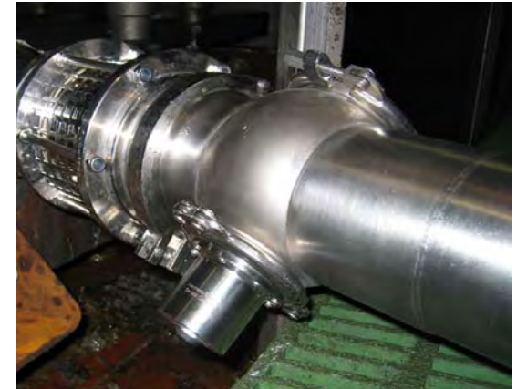
Sensor installed in pipe
